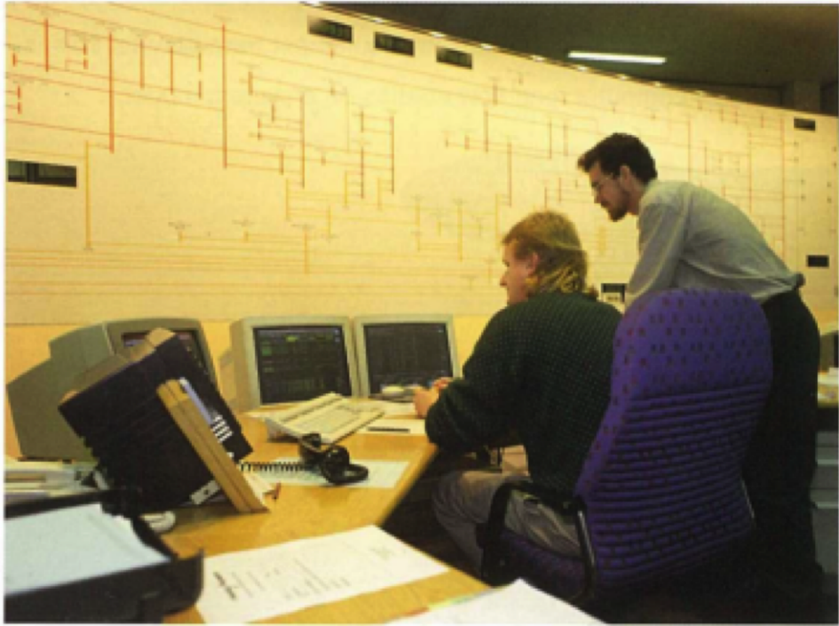
Figure 10: The System Operator control room for the North Island Grid, circa 1995 (the author is the one standing). From information booklet Trans Power Control Centres produced in 1995 (when Transpower was written as two words).
