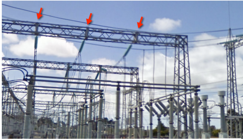
Figure 6: Otahuhu substation with the three phases of the 220kV bus indicated (this picture is from Google Street View).
